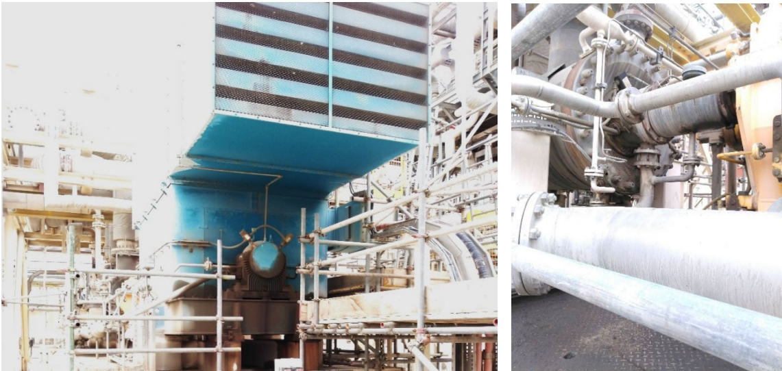
Figure 4. Lubrication System Failures
