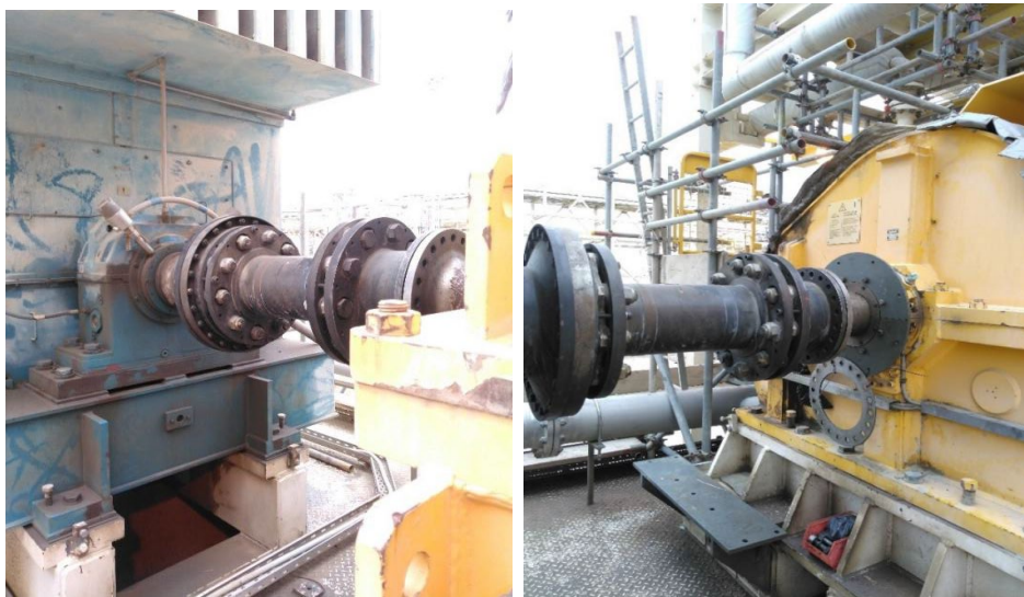
Figure 3. Gearbox and Compressor Shaft Transmission Coupling
