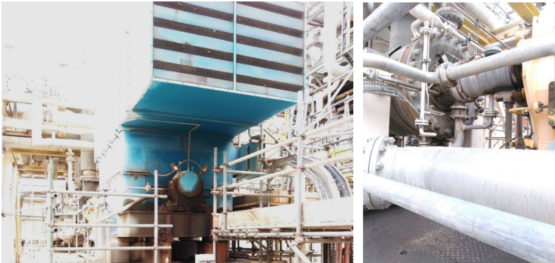
Figure 4. Lubrication System Failures
