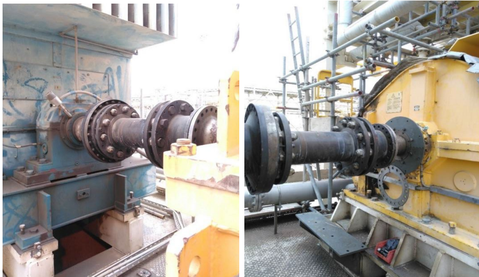
Figure 3. Gearbox and Compressor Shaft Transmission Coupling
